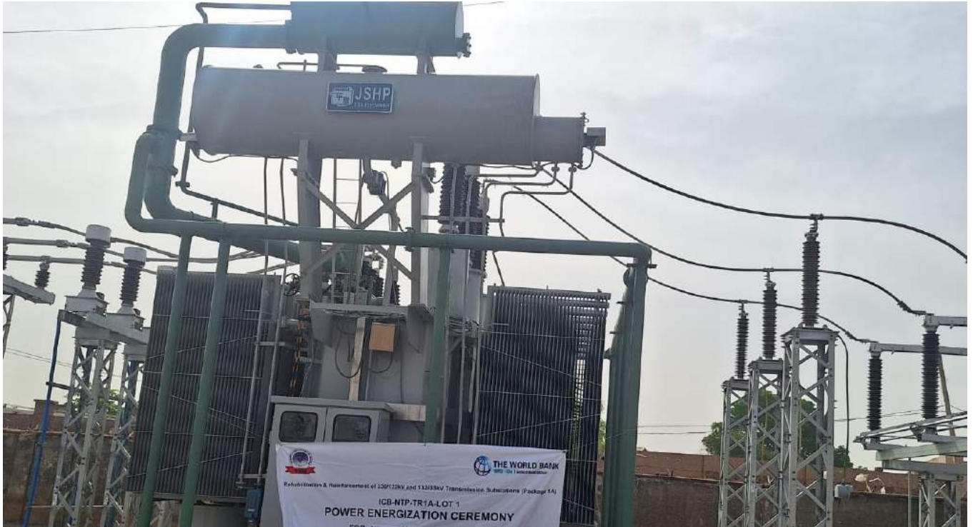
100MVA 132/33kV power transformer at Dan Agundi Transmission Substation
