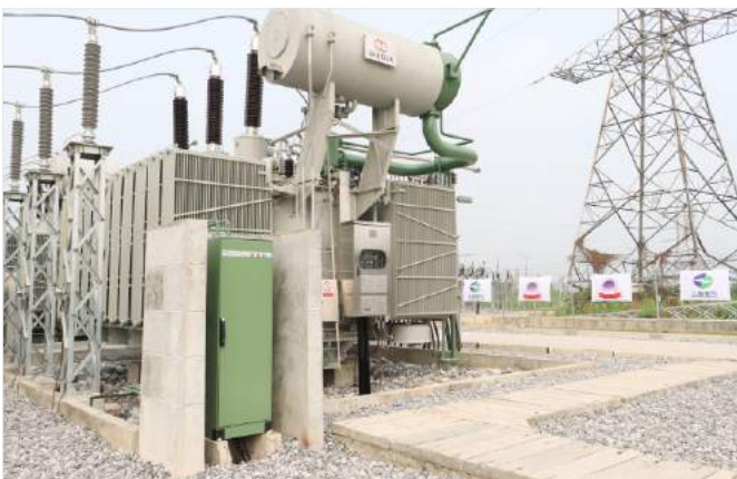
Side view of one of the transformers
