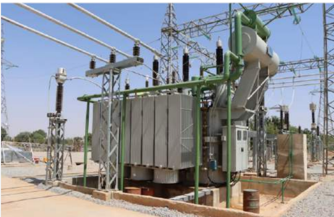
The newly commissioned 60MVA power transformer at 132/33kV Kankia Transmission Substation, Katsina State
