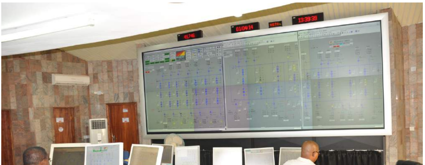
Control Room at NCC,Osogbo with mimic board display
