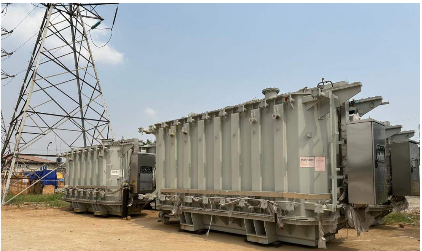
Some of the transformers delivered to Akangba Transmission Substation, Lagos State
