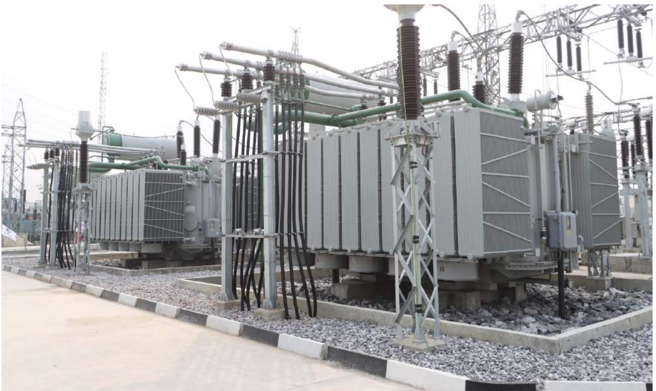
The 2x100 /125MVA Power Transformers commissioned at Alagbon Substation
