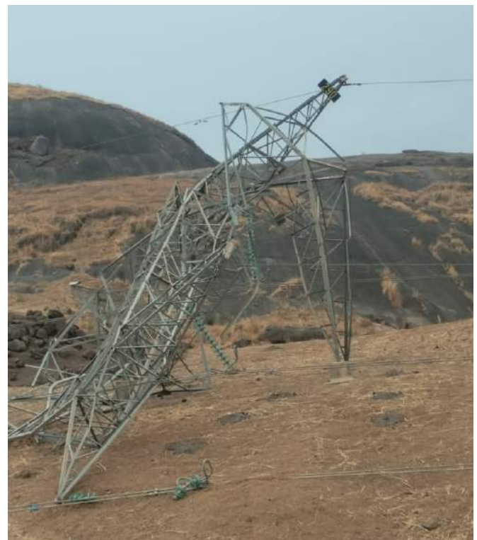
One of the four towers vandalised along the Jos - Gombe 330kV Transmission Line
