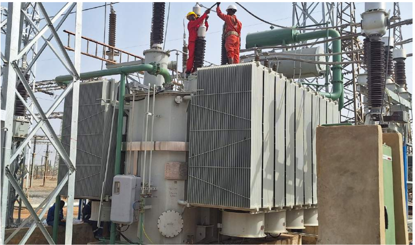
The energised 100MVA power transformer at 132/33kV Dakata Transmission Substation, Kano State
