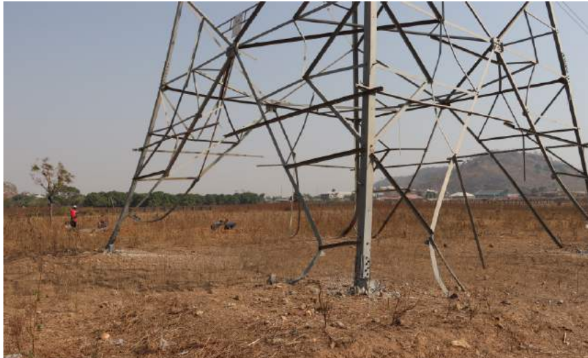
Loosened bolts on a tower
