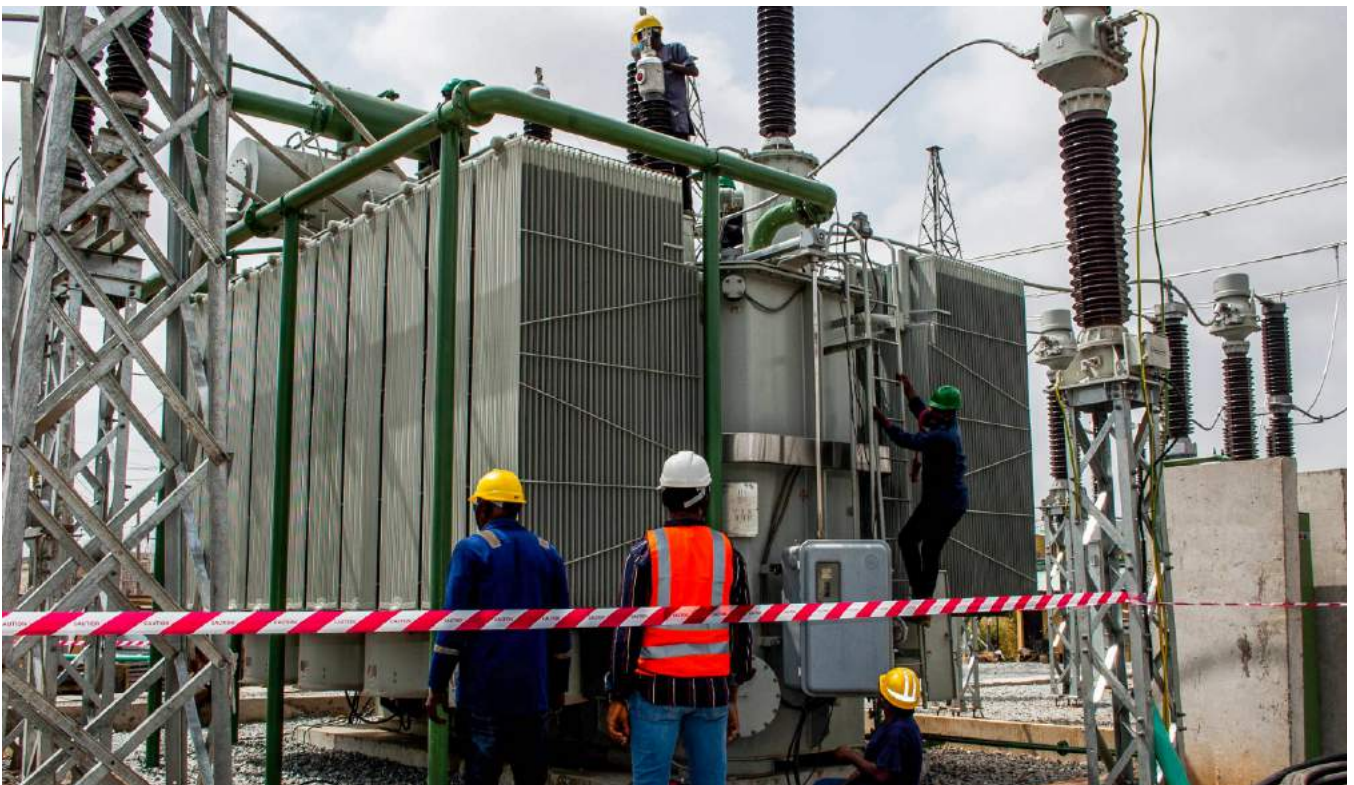
Commissioned 100MVA power transformer in 132/33kV Ganmo Transmission Substation, Kwara State
