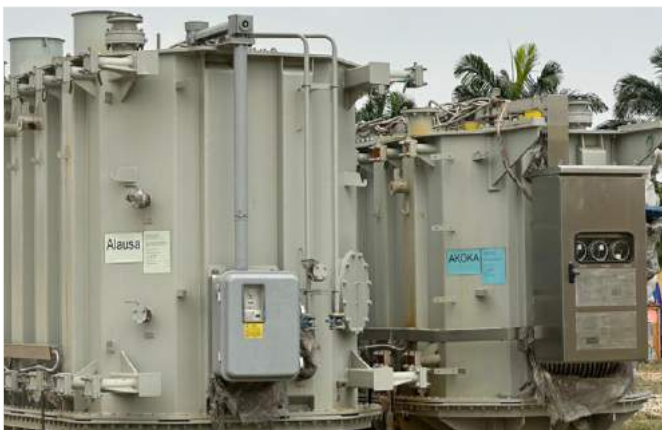
Side view of some of the transformers
