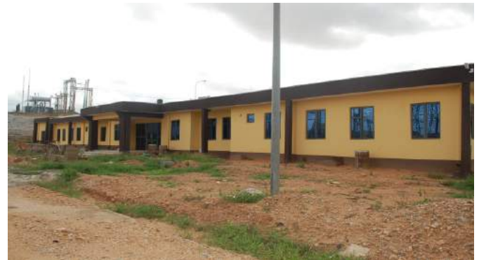
Ongoing Construction of New Office Complex for Staff at Ayede Transmission Substation
