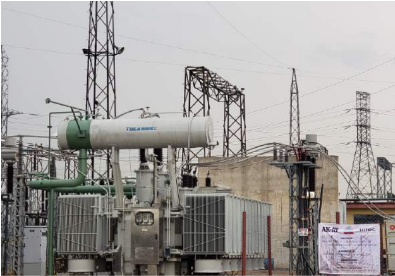
Commissioned 100MVA Power Transformer at Port Harcourt Main Transmission Substation
