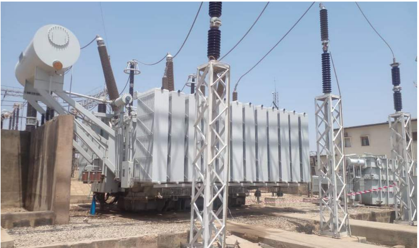
The newly commissioned 150MVA power transformer at the 330/132/33kV Jos Transmission Substation
