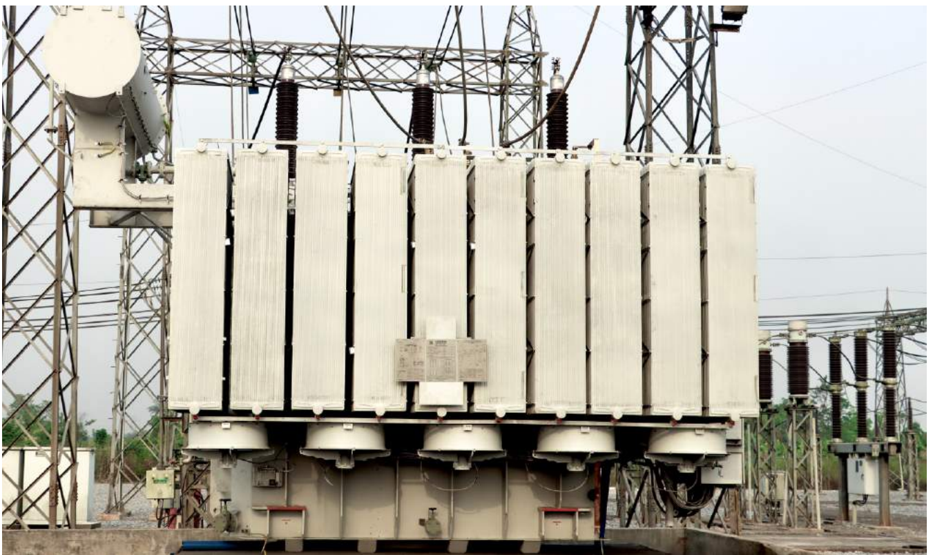
The 100MVA power transformer commissioned at 132/33kV Ihovbor Work Centre, Edo State
